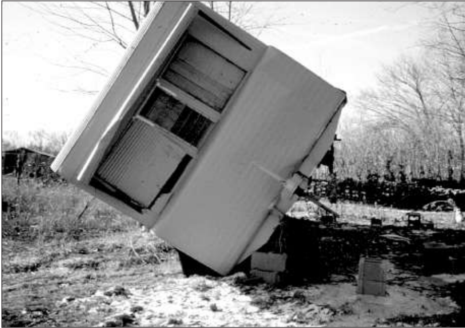
Figure 7-8. Failed foundation system that used masonry piers.
