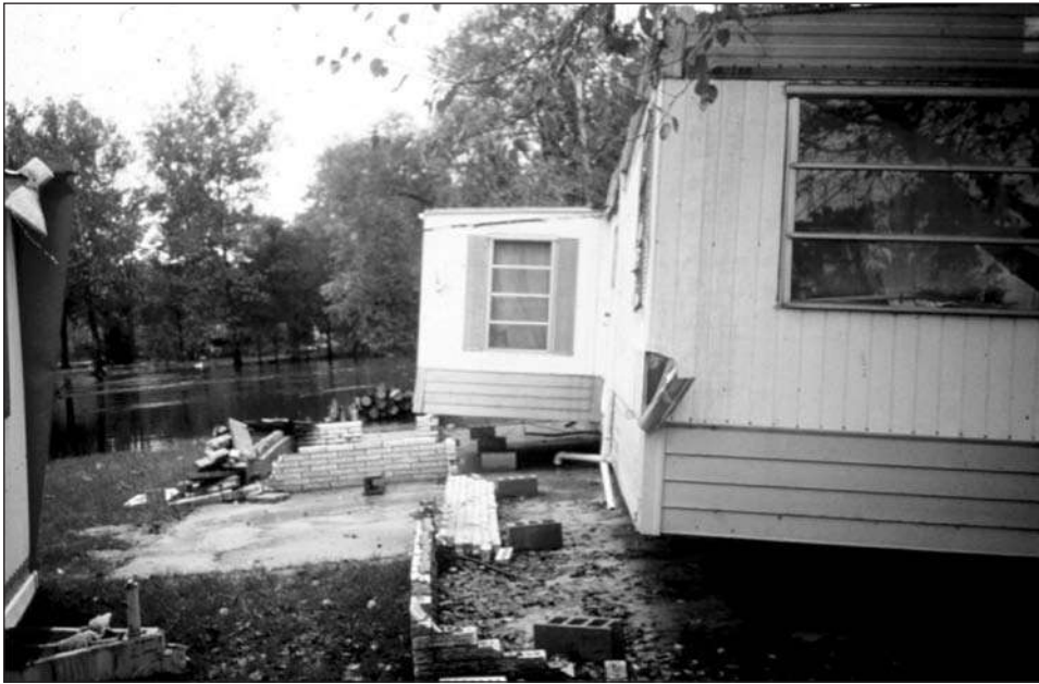
Figure 9-1. A home that was partially submerged and displaced from its foundation by hydrostatic forces. Although it appears the openings are too high, the bottoms of the openings are less than 1 foot above the top of the interior slab.
